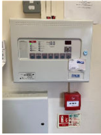
Woodhouse CC Fire Panel
