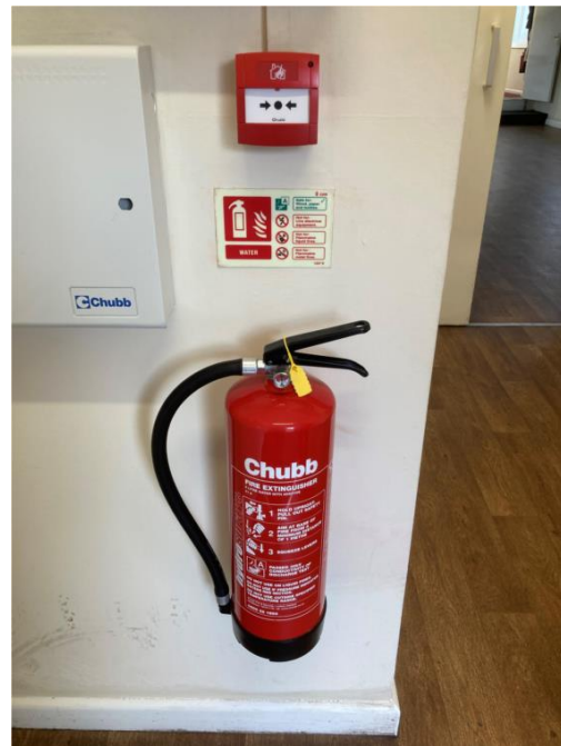
Woodhouse CC Identified Extinguishers
