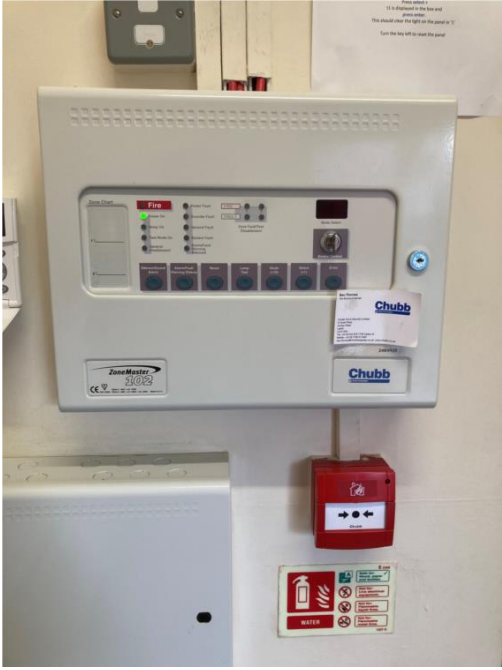
Woodhouse CC Fire Panel
