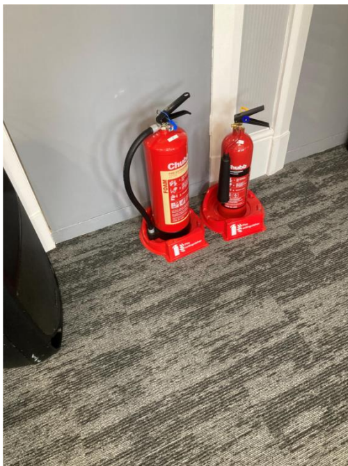
Identified Fire Extinguishers
