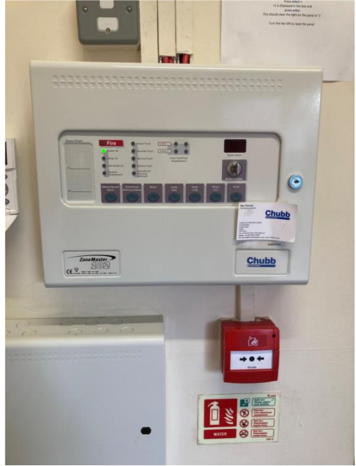
Woodhouse CC Fire Panel
